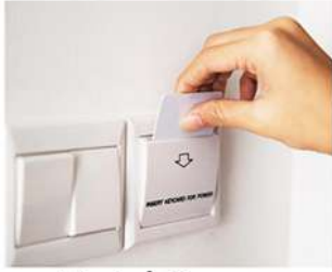
Hotel Room Occupancy System
